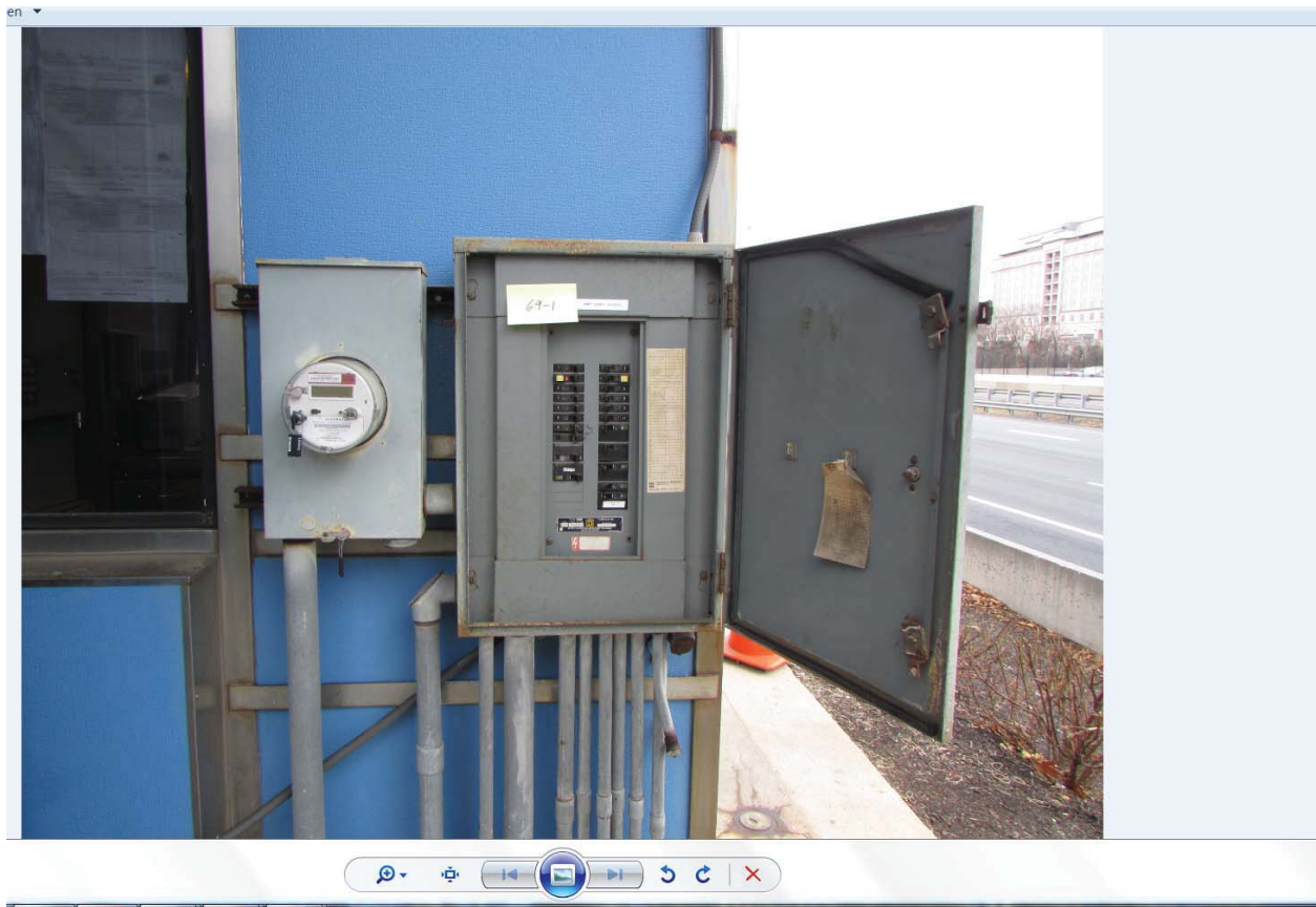
Figure 1.0 C Typical Condition inside Panelboards
